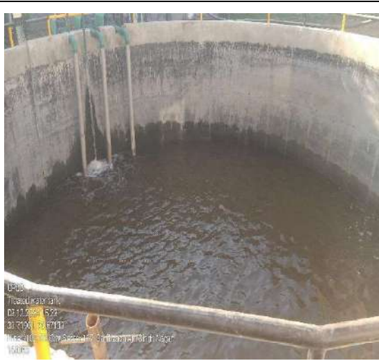
Treated Water Tank of 2.5MLD STP, TDI, Sector 117, Mohali
