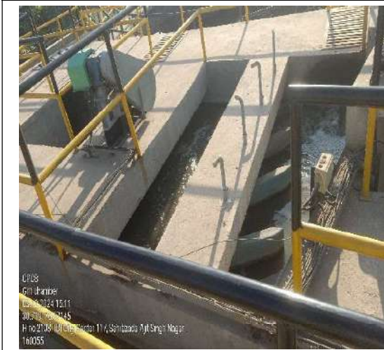
Grit Chamber of 2.5MLD STP, TDI, Sector 117, Mohali
