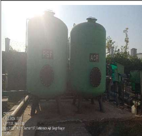
PSF & ACF (Filters) of 2.5MLD STP, TDI, Sector 117, Mohali
