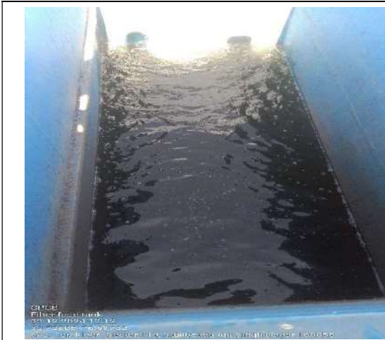
Filter feed tank of 100 KLD STP, Sector 119, Mohali
