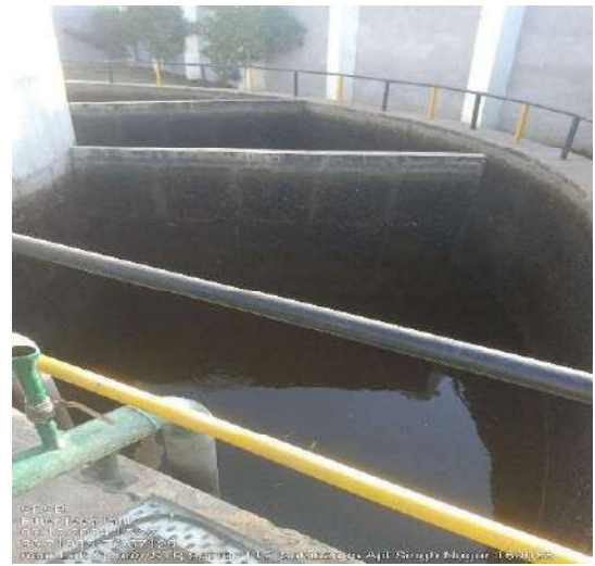
Filter Feed Tank of 2.5MLD STP, TDI, Sec. 117, Mohali
