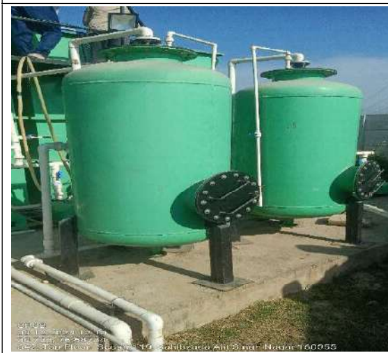
PSF & AC Filters of 100 KLD STP, Sector 119, Mohali
