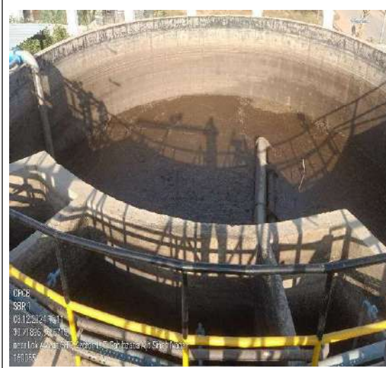
SBR Tank 02 of 2.5MLD STP, TDI, Sec. 117, Mohali
