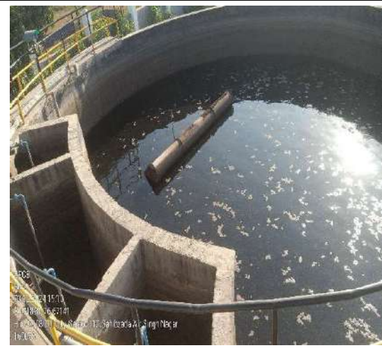
SBR Tank 01 of 2.5MLD STP, TDI, Sec. 117, Mohali
