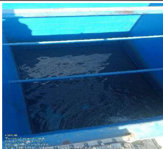
Treated water tank of 100 KLD STP, Sec. 119, Mohali
